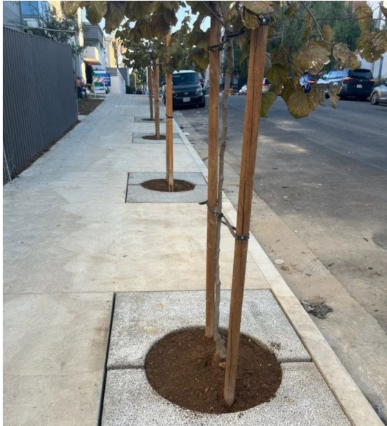
Source: Pacific Pervious Concrete
